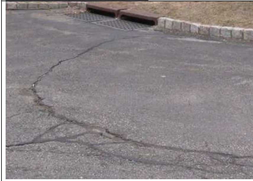
Photo # 9- parking lot is worn, settled, large cracks and in need of patch work, top coat sealing and continued maintenance. This also lends its self to "curb appeal" for a business or complex.
