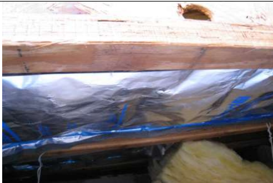
Photo # 23 & 24- Partial view of roof structure as viewed on ladder at roof scuttle opening peering through acoustic ceiling tiles. Insulation, was installed between decking and acoustic tiles (below-not visible in picture). Some black iron gas pipes, electrical and ductwork visible and covering framing.
