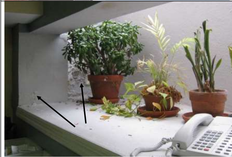
Photo # 52- Efflorescence, peeled paint; indication of water intrusion
