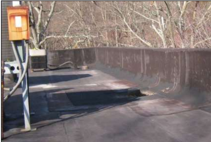
Photo # 4 - Two of the three internal roof drains along the north parapet wall. Notice scupper drains were sealed. See next picture #2
