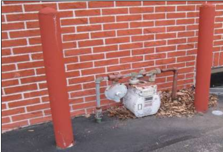
Photo # 10- Crash barriers are close to the gas meter and building not affording optimal protection against accidental vehicle contact from oblique angle. Recommend a third barrier in front and between existing barriers.
