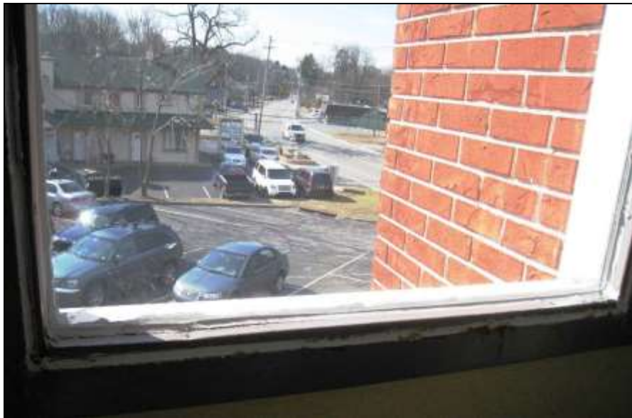
Photo # 16- Heavy caulking and rust around inside of older windows. Recommend proper repairs or replacement.
