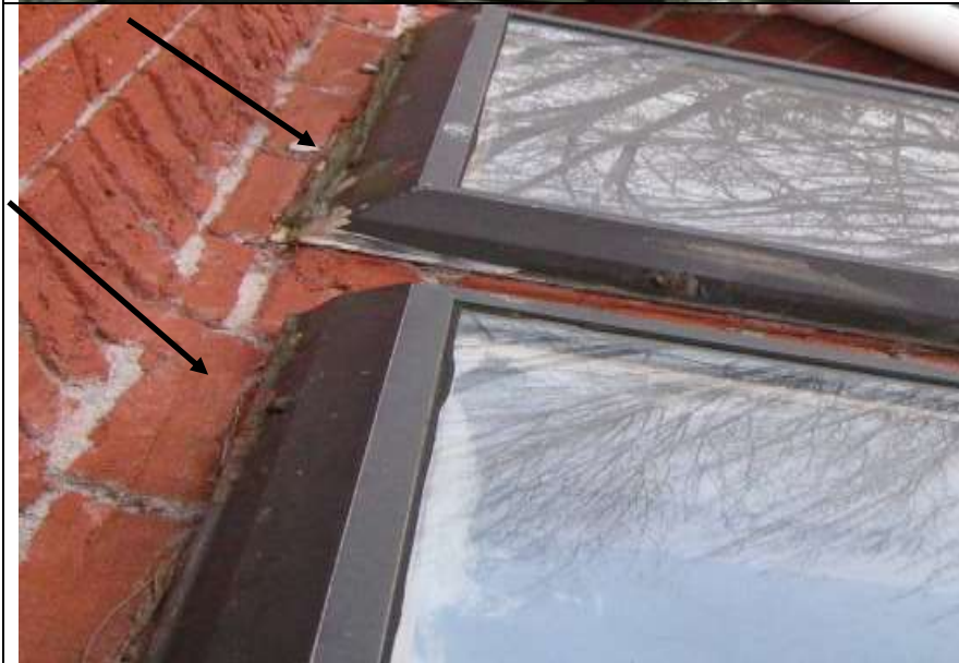
Photo # 51- Heavy caulking around skylights. Cracks, gaps and sprayed expansion foam visible from interior kitchen
