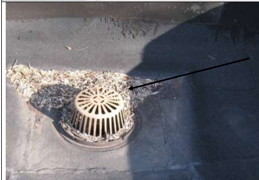
Photo # 26- Debris in depression around drain. Monthly inspections are recommended and cleanings to keep clear for proper flow.
