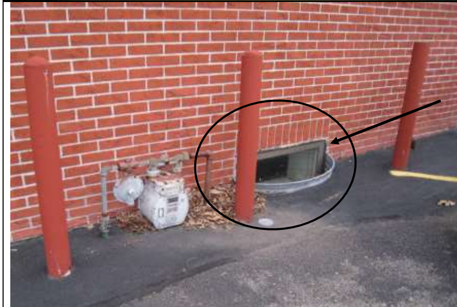
Photo # 17- No window well cover installed. Rain, ice and snow will collect in well and infiltrate into basement.
