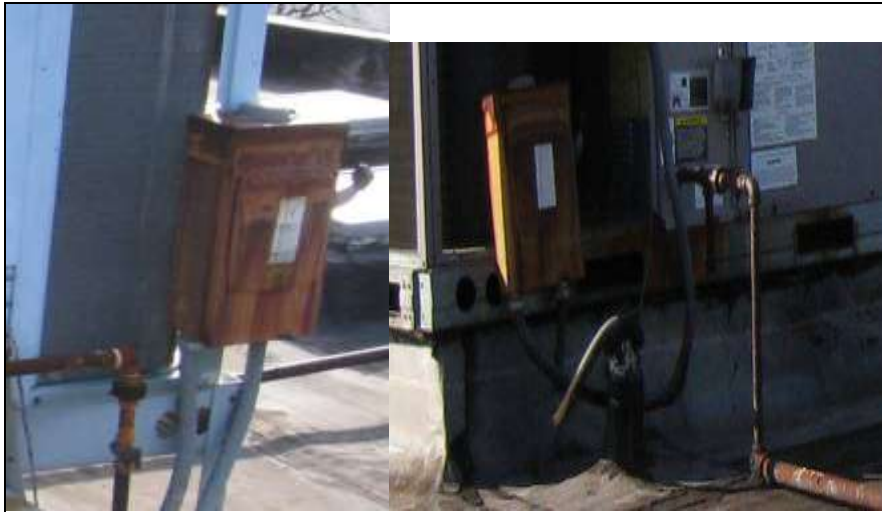
Photo # 22- Typical of the rusted disconnects on all RTU's and A/C compressors. Rusted black iron gas lines and fittings.
