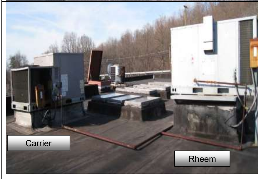
Photo # 18- East side roof, Carrier (left) ~10yrs old and Rheem packaged unit (right) 2004 manufacturing date on unit. Units have very rusted gas supply lines and disconnects.
