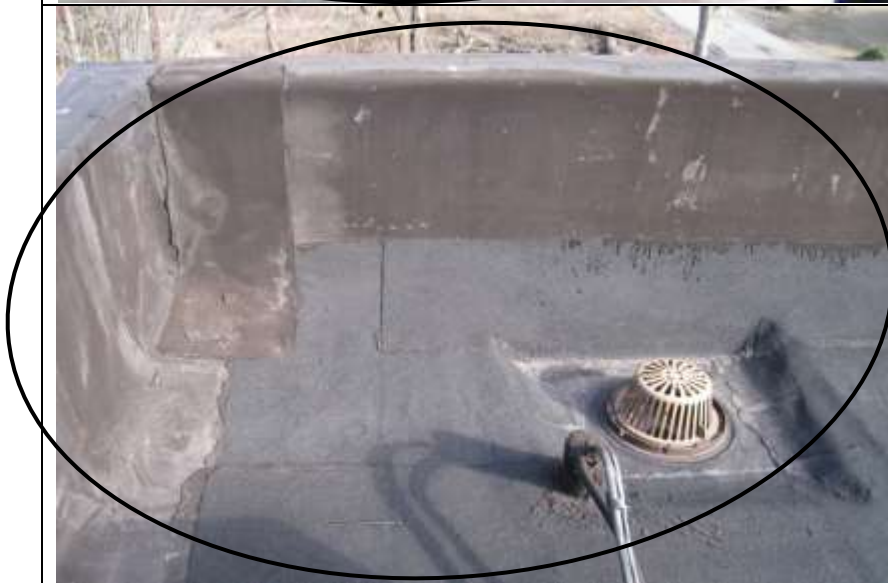
Photo # 29- Membrane and asphalt rolled roof patching around internal roof drains and parapet wall
