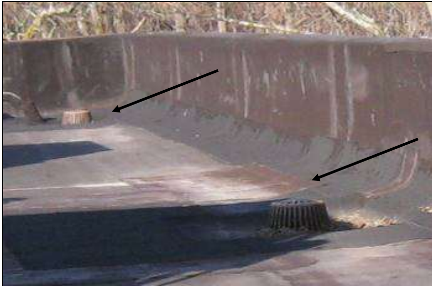
Photo # 25- two of three internal roof drains. Heavy patching along the base flashing on north wall.
