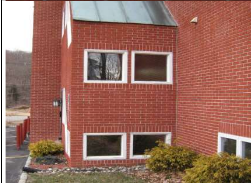
Photo # 6- Copper roof drains onto ground below where stones and black drainage tiles is positioned. Drainage tile has flat pitch and tips upwards toward curbing. Drainage is not adequate and water tends to collect against foundation. Consider adding gutter and rain leader to improve water drainage.
