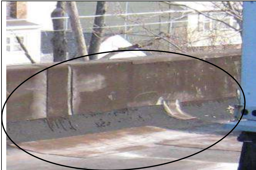
Photo #28- Numerous patching along north wall
