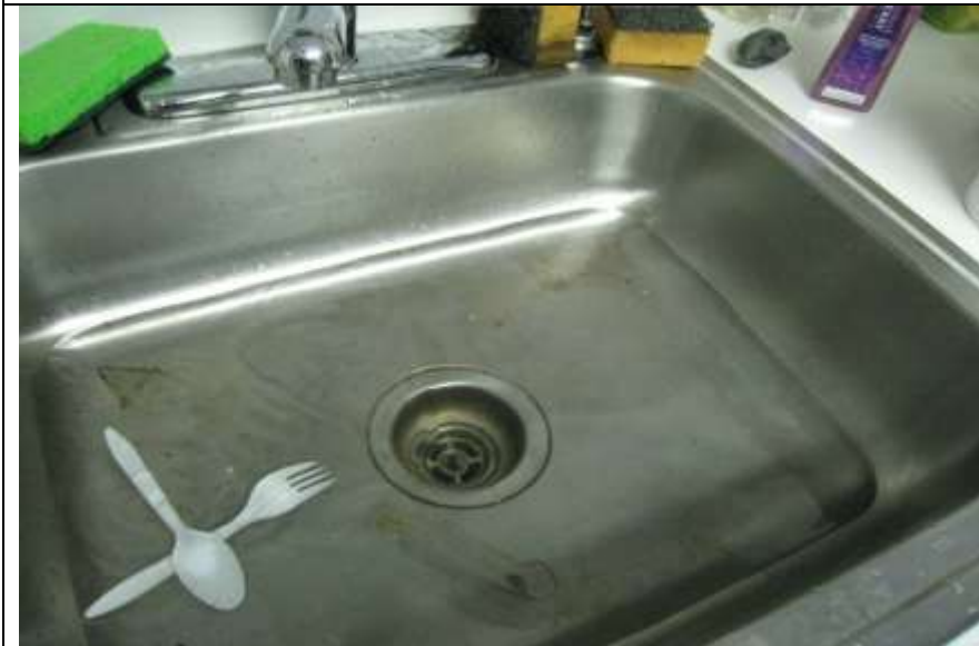
Photo #49- Kitchen sink in basement (Promotional company Suite). Sewer ejector pump was running and water did not drain properly.
